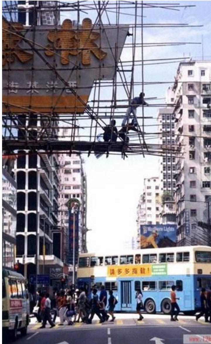
Chinese scaffolding. Just how safe is it!
