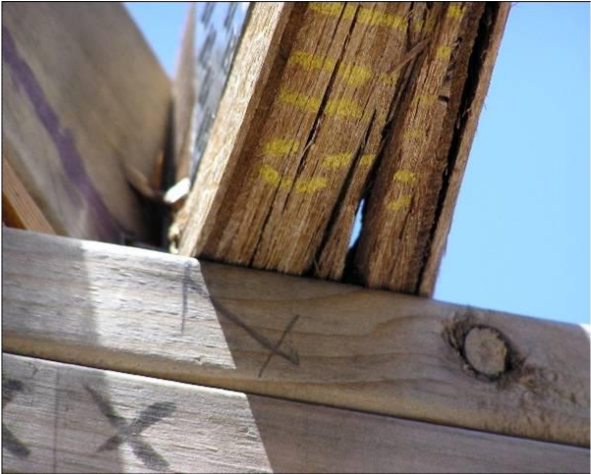
Poor showing: Severe delaminating in a Chinese LVL product imported into Australia.
